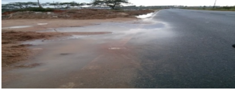
Fig. 9: Improper Construction of Shoulder and Water Stagnates along the Network
