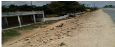
Fig. 10: Absence of Culvert Near Depressed Build-up Area
